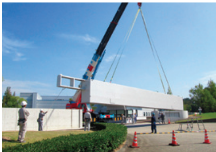
Otsuka Pharmaceutical Factory: Full-circumference seawall installed at Matsushige Factory
